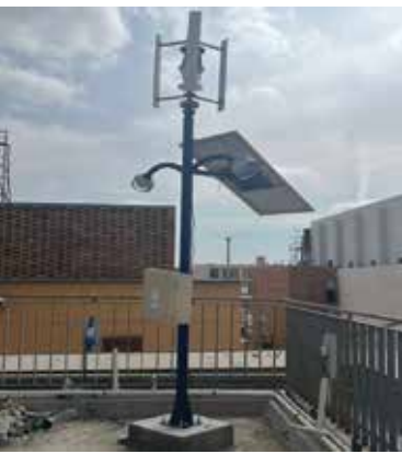
Street lighting using Solar wind energy students' graduation project
