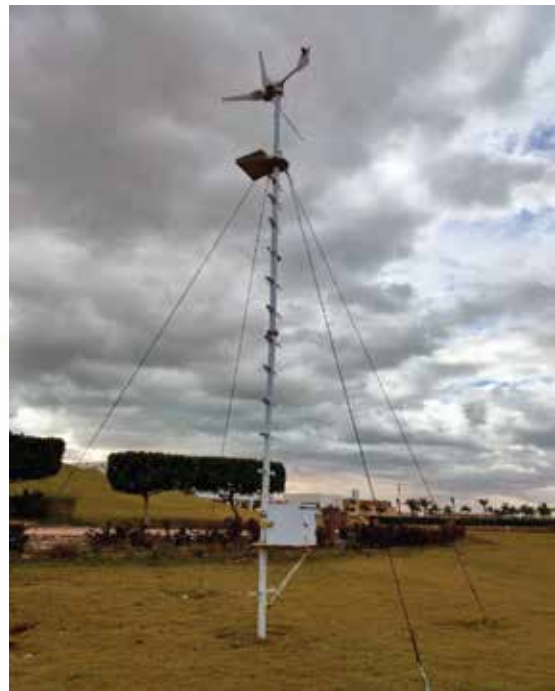
Wind energy power generation at EJUST
