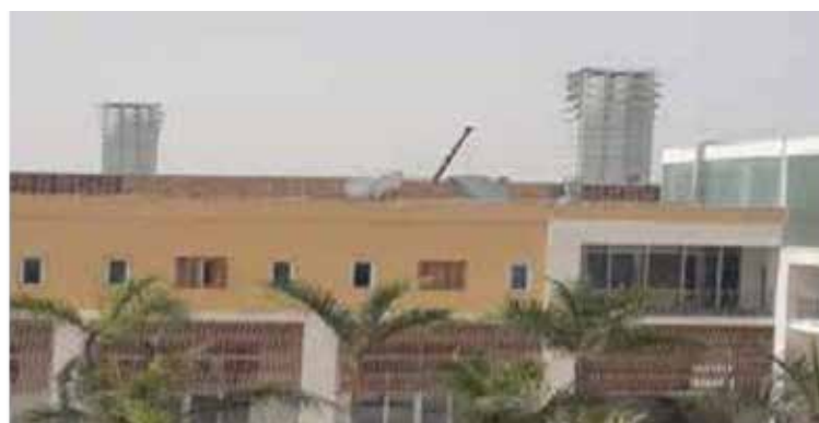
EJUST ventilation system
